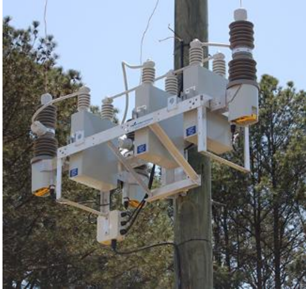
Pole-Mounted Capacitor Banks
