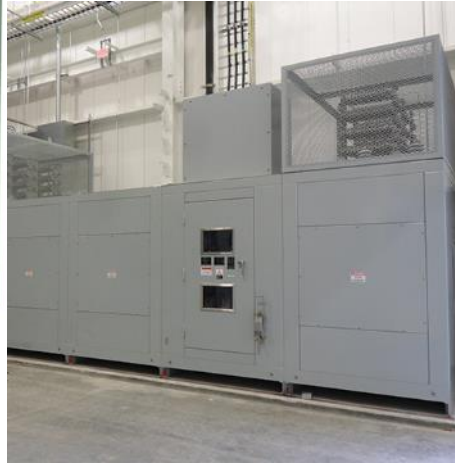
Metal Enclosed Capacitor Banks
