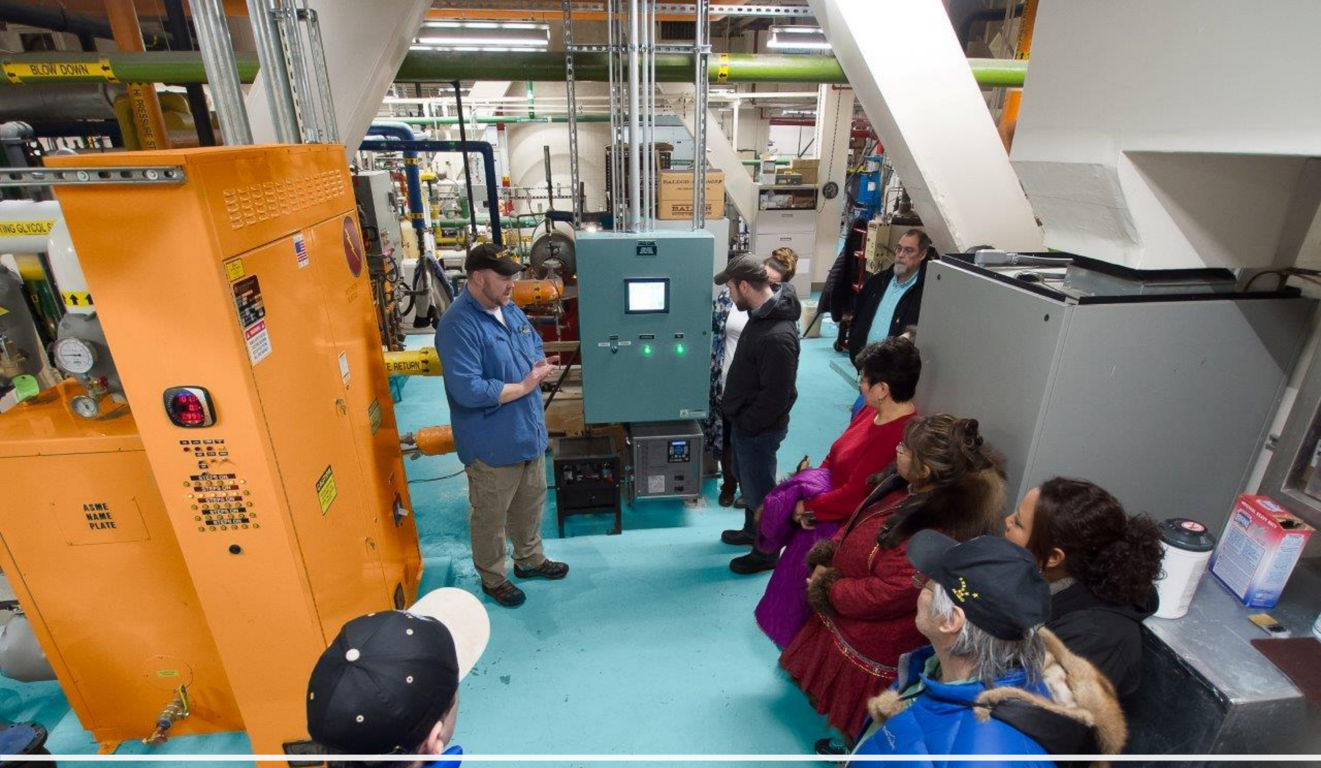
Hospital 450kW Electric Boiler (first B/E Project in 2016)
