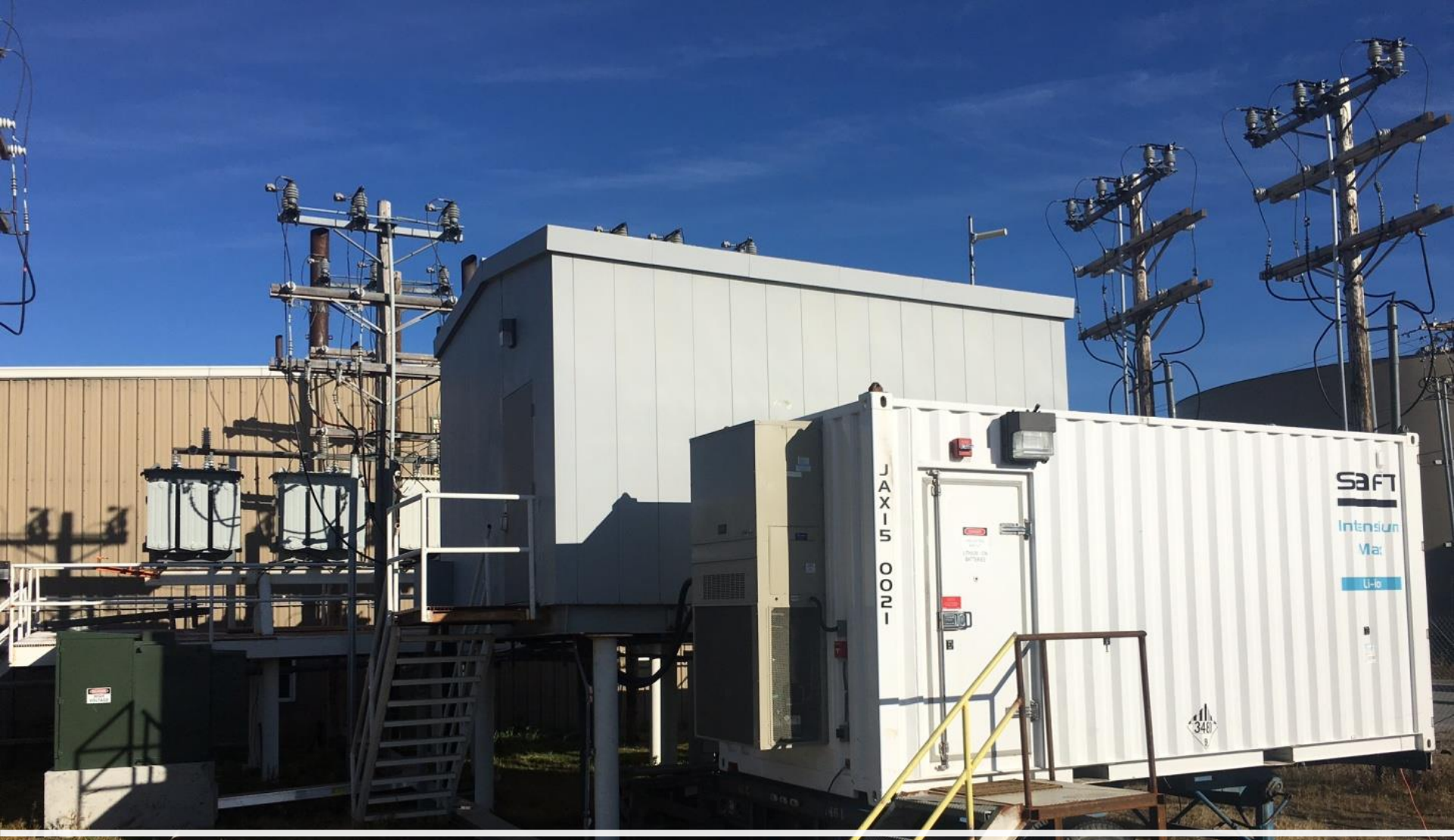
SAFT 950 kWh Battery (ABB 1.2MW Inverter in Plant)
