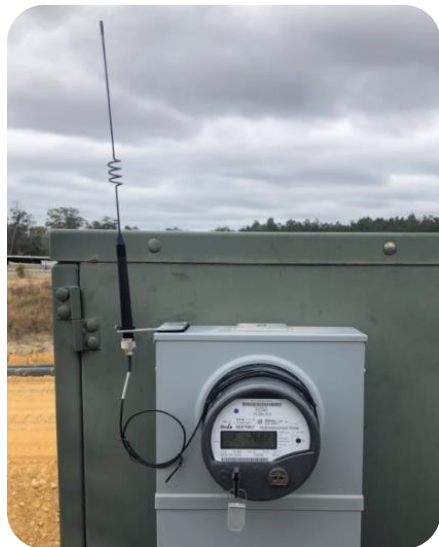
Passive Coupled Meter Antenna
