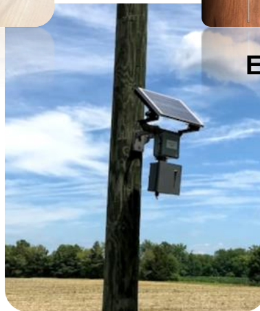
Solar Power Supply
